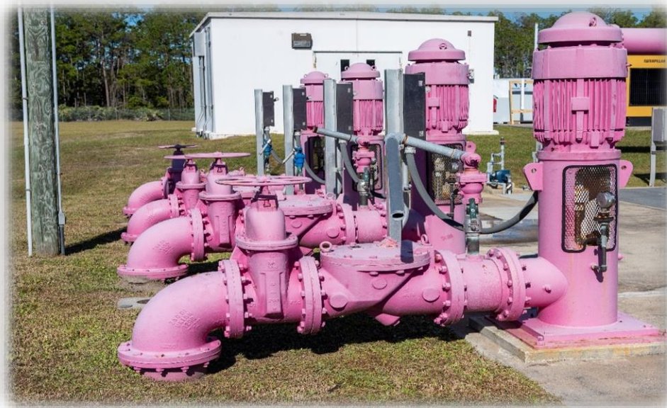
Reclaimed water pumps at the Fleming Island Regional Wastewater Plant in Clay County.
